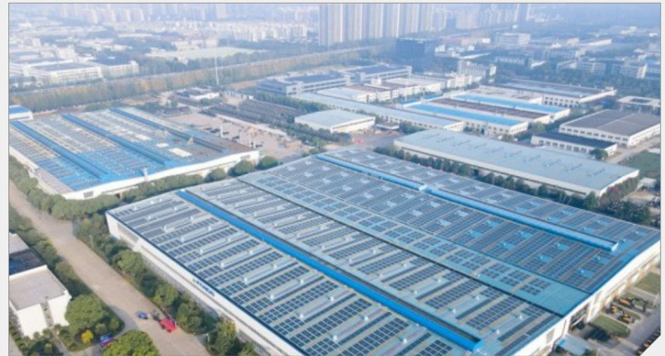
4MW rooftop solar installation at the subsidiary in China
