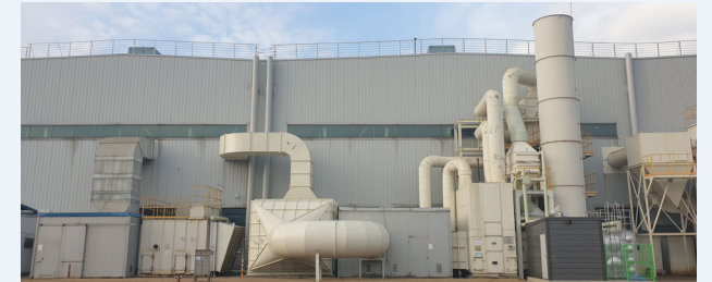
Heat Exchanger for Waste Heat Recycling at the Gunsan Plant
